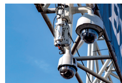
CCTV & Visitor Counting Solutions
